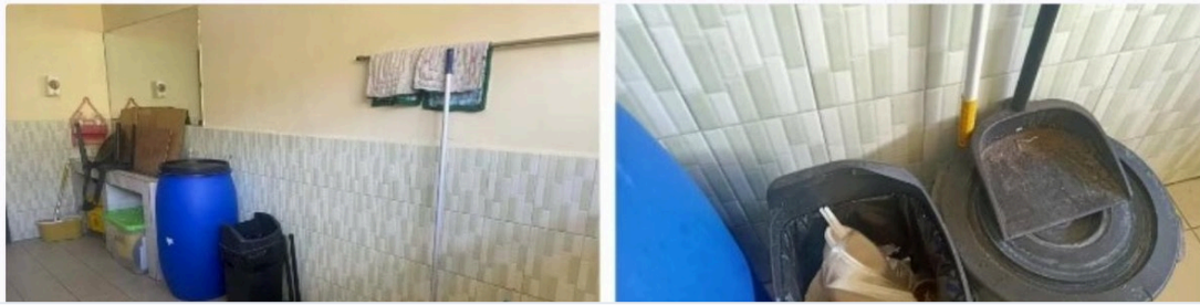
FIG. 2 Field inspection photographs of IBIS Senior High School restroom facilities: storage items occupying toilet areas, broken fixtures, graffiti on walls, improvised partitions, and urinal sections in disrepair. These conditions document the cleanliness and usability gaps driving the 3.43 weighted-mean satisfaction rating across 89 student respondents.
